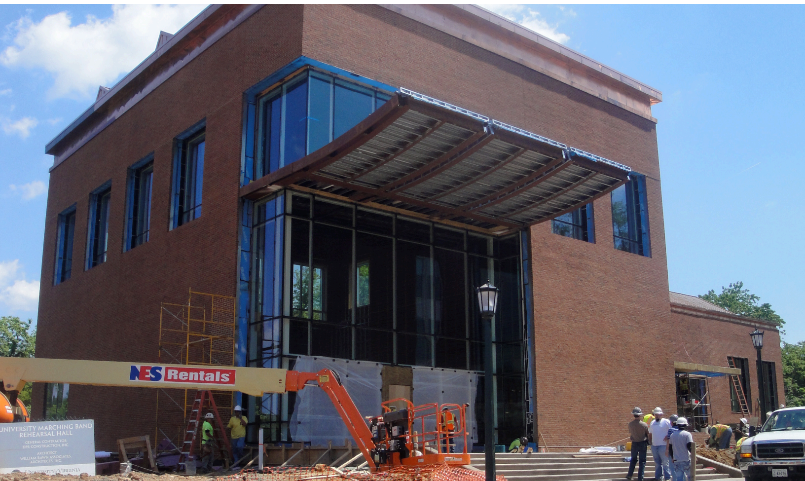
BELOW: The $10.7 million Hunter Smith Band Building nears its completion in the Casteen Arts Grounds
